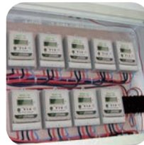
Power Distribution Panels
